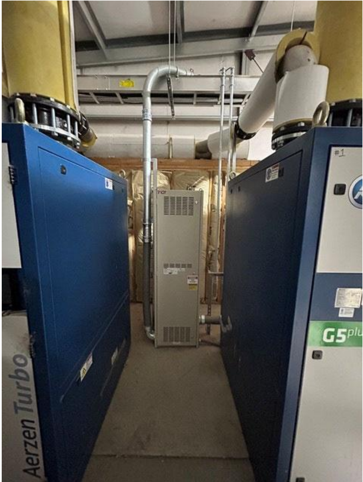
PHOTO OF EXISTING TURBO BLOWERS #1 AND #2
