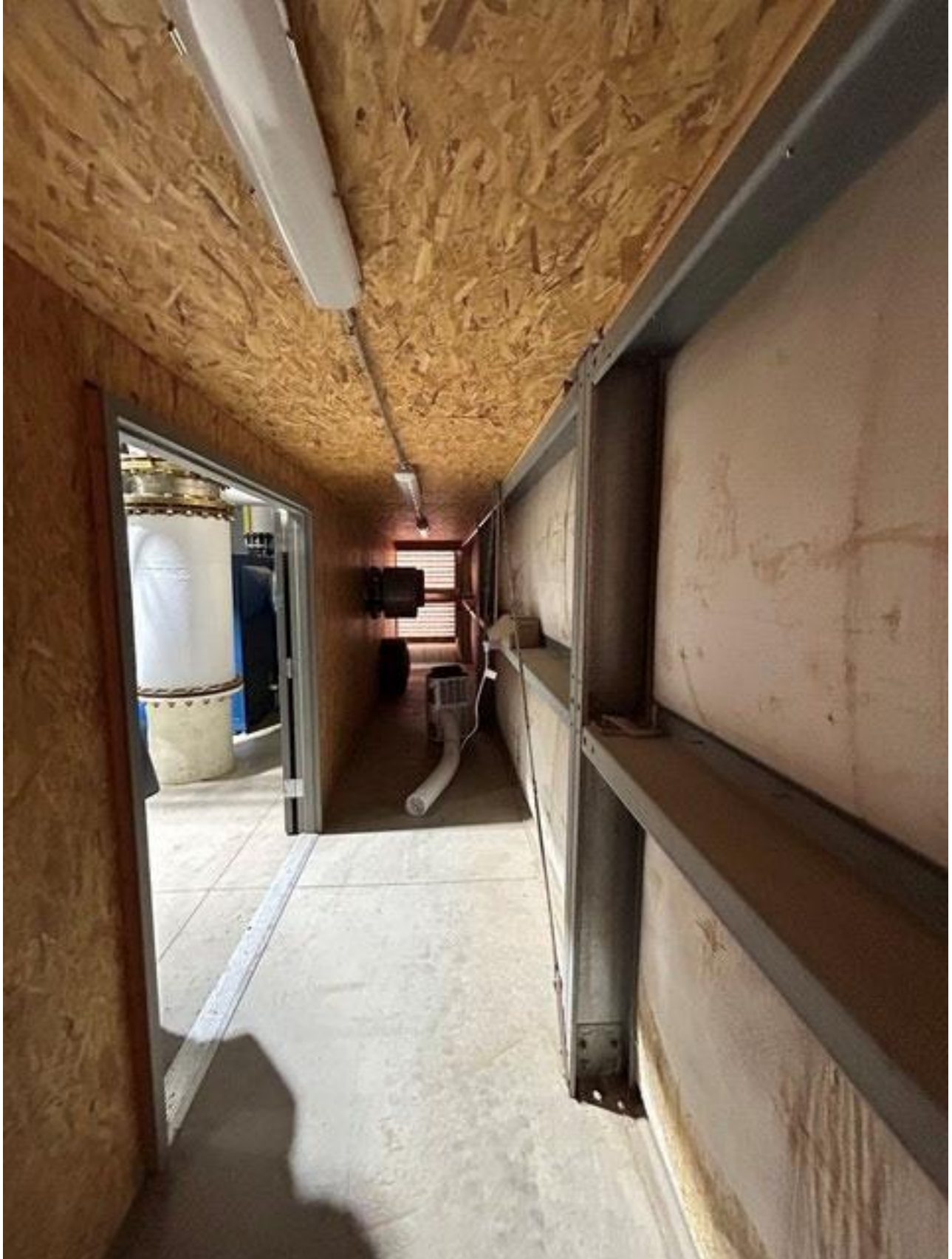
PHOTO OF PLENUM ROOM
