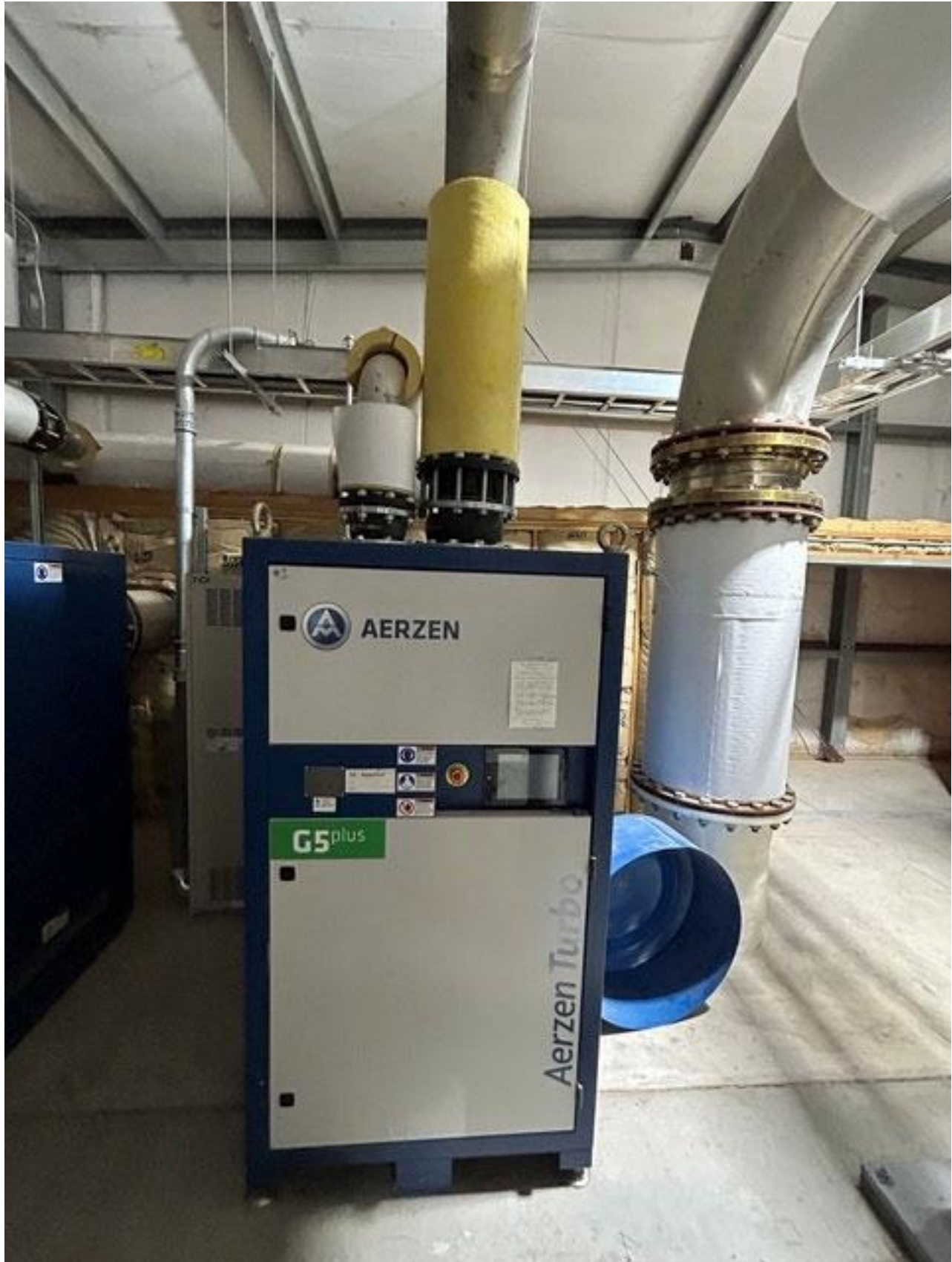
PHOTO OF EXISTING TURBO BLOWER #2
